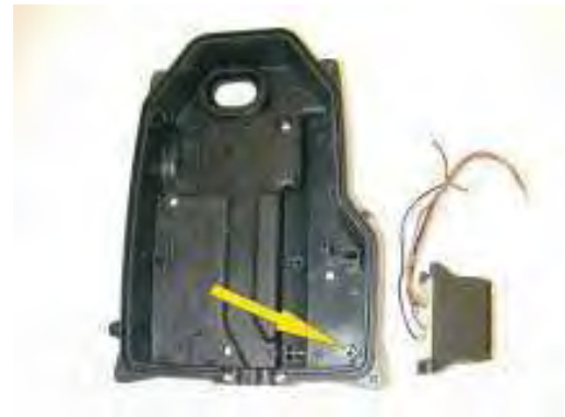
Fig. 6: Electrical box with old transformer
