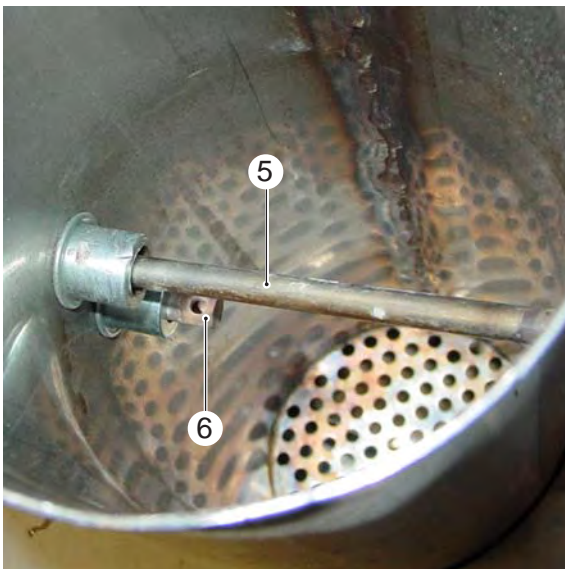
Measuring points in the exhaust connecting sleeve
