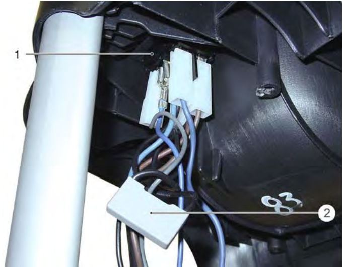
1 Main switch for brushing/vacuuming operations 2 De-interference capacitor
